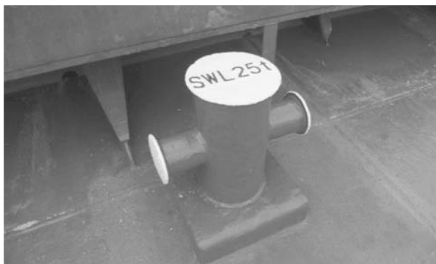
Cruciform Bollards on Tankers in the Manifold area
