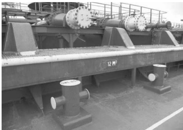
Tankers Cruciform Bollards in the Manifold area
