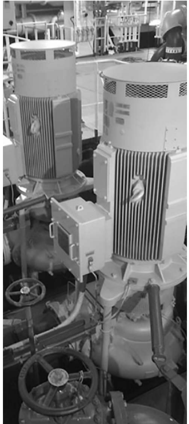
Figure 5. Two ballast pumps of 1,500 m 3 capacity on a container vessel
